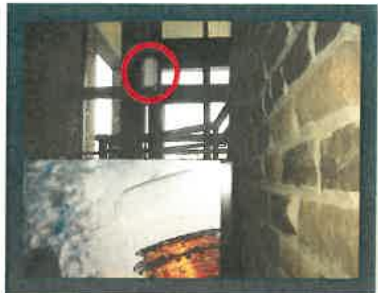
The photo above shows an installed vending miser.
