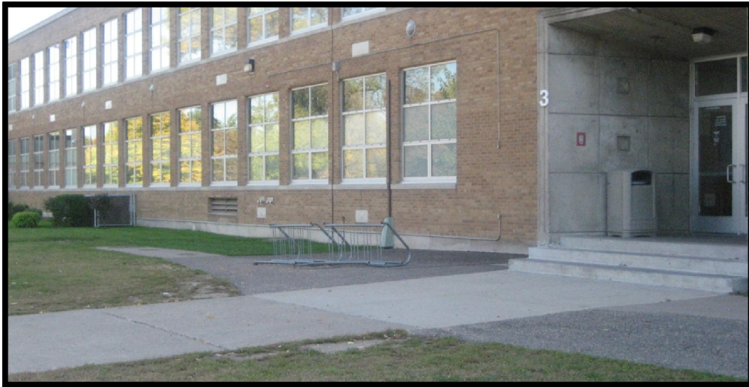
Two bike racks located near Door 3, on the north side of the school.
