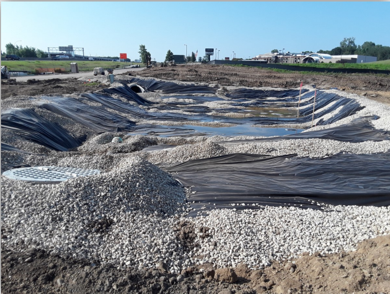
(Above) The pretreatment cell was sized for increased capacity and native soils were replaced with an engineered mix meant to enhance infiltration.
