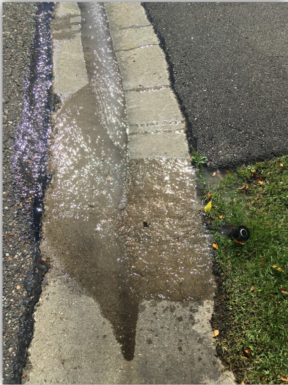
(Left) Significant runoff is observed next to a broken rotor.
