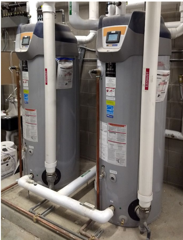
Image of hot water heaters
