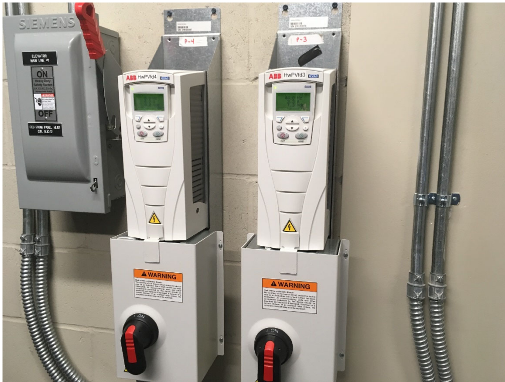
Image of pump VFDs
