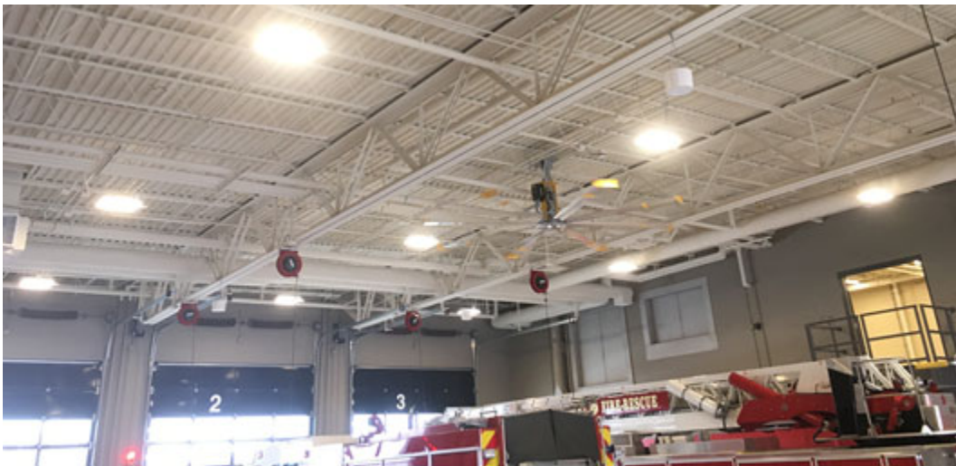
Image of Apparatus Bay lighting
