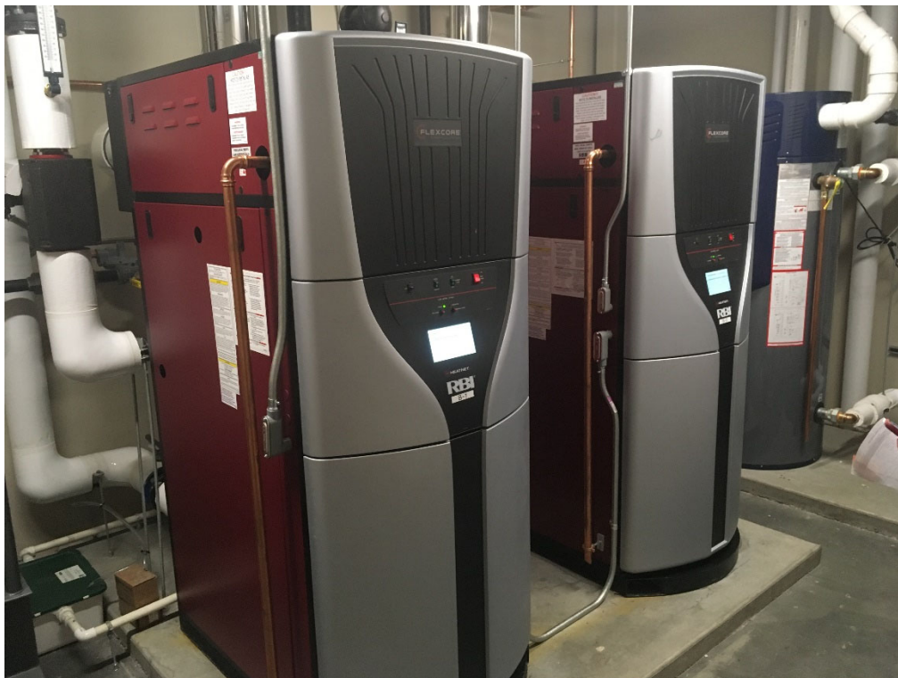
Image of boilers
