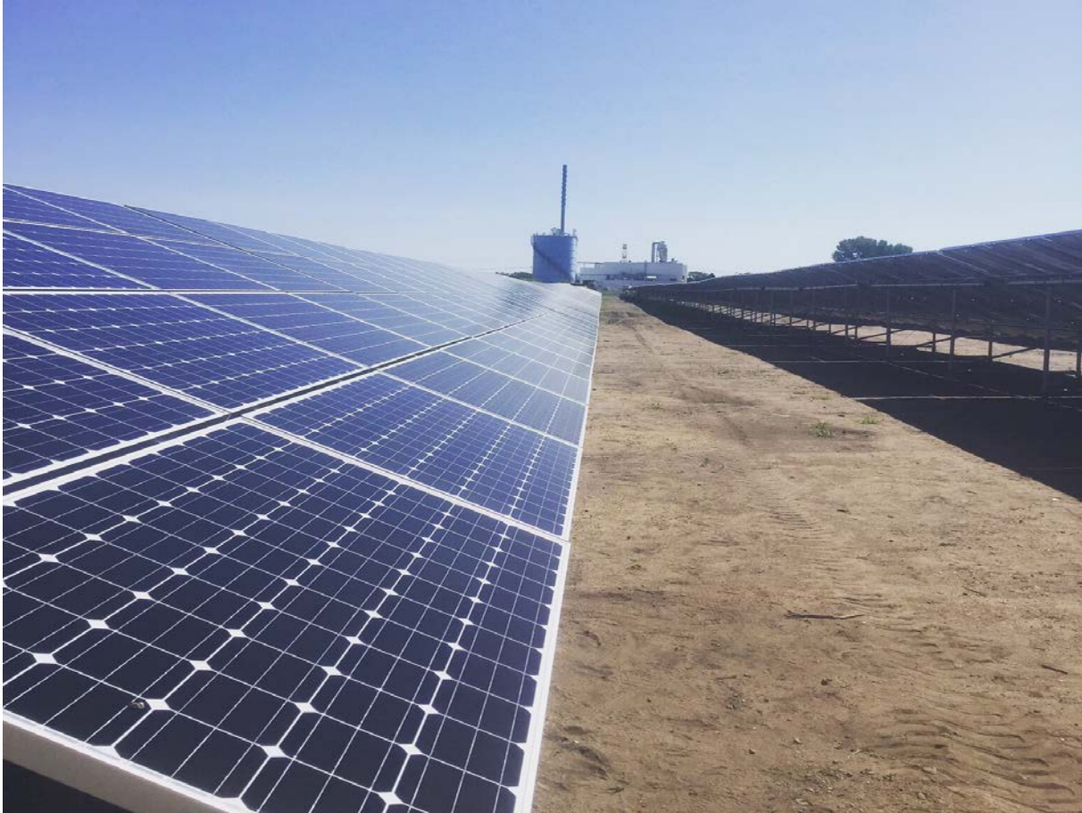
Blue Lake Solar Facility: Looking east at the Blue Lake WWTP
