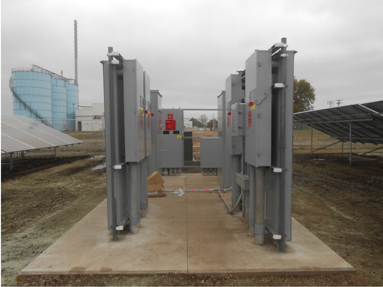
Equipment Pad: Looking east towards Blue Lake WWTP
