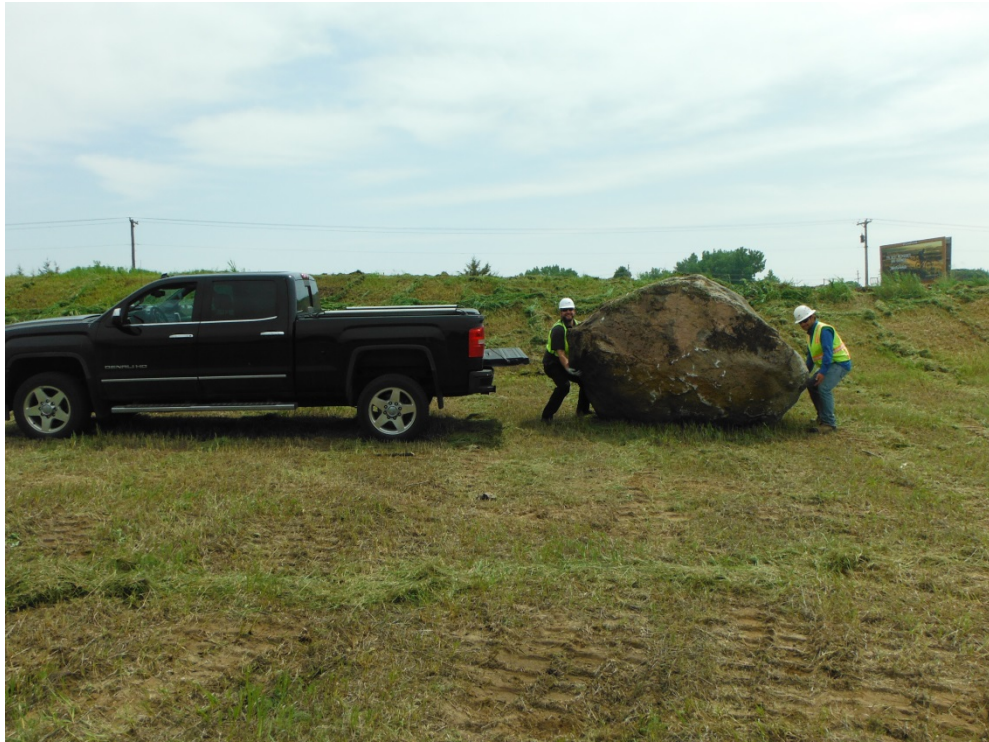
An example of bedrock encountered during site preparation at the Blue Lake solar facility
