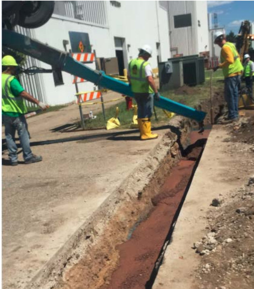
Medium Voltage interconnection wires encased in concrete on the Blue Lake WWTP property
