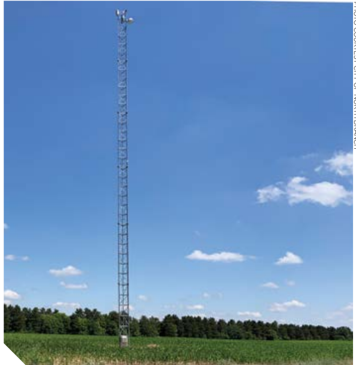
This is one of three towers that serve the new broadband network.
