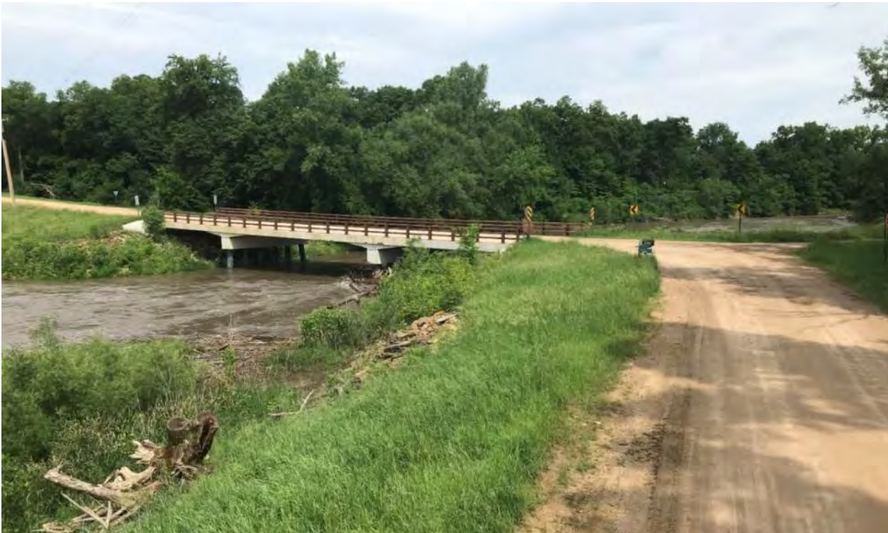
Figure 17: Stream bank on Ivy Road on Maple River Restored after September 2010 Flood
