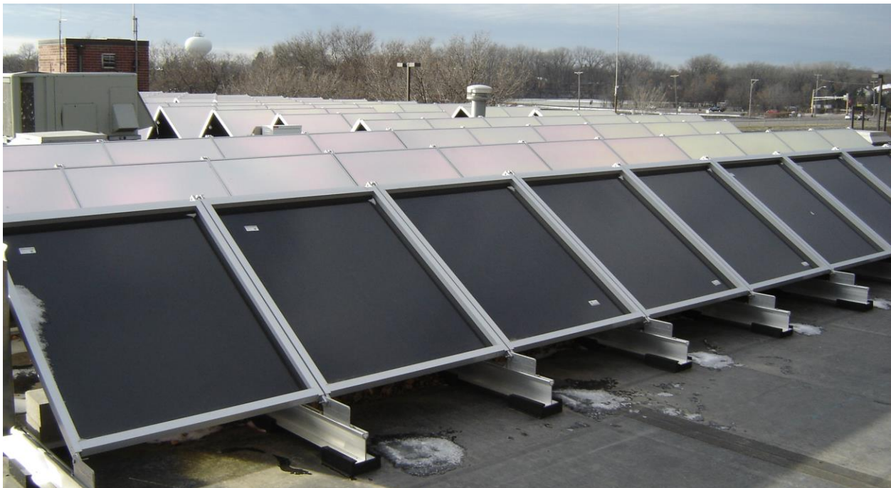
Solar Panels atop City Hall. Photo Credit: City of Falcon Heights.
