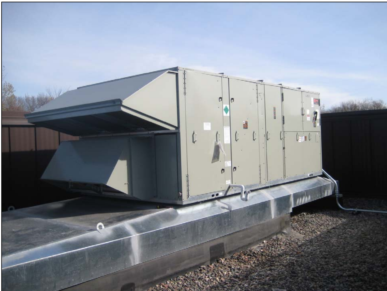
New Rooftop Unit for City Hall/Police
